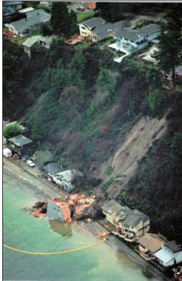
Figure 29: Landslide in Rolling Bay occurred after a hundred-year rainstorm in Dec, 1996 (Seattle Times).
